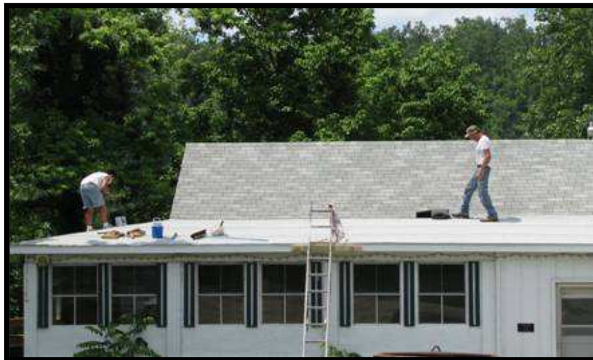
Randy and Stephanie Pendgraft of Improvements R Us (870-404-9940) replace a portion of the Spring House Roof
